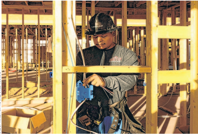
Raul Guzman installed electricity in a new home in Surprise, Ariz., last week.
